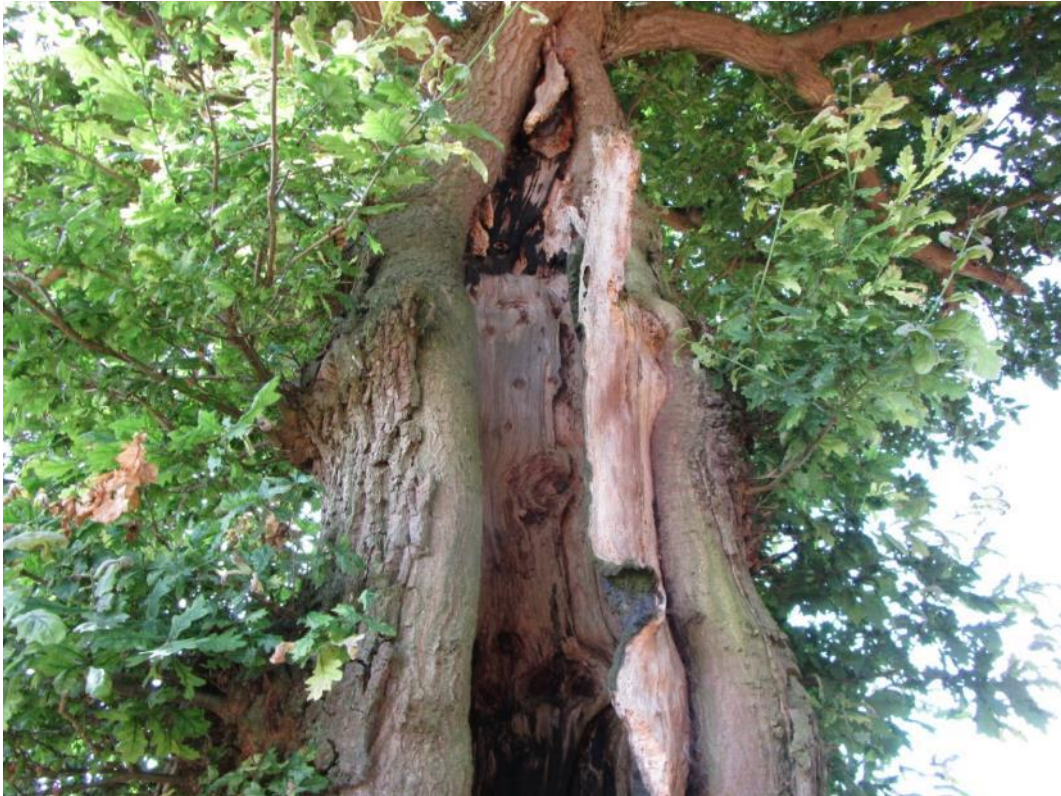
9: Decay on a hollowed-out Quercus [oaks] tree just outside the proposed Bypass Route [B8]
